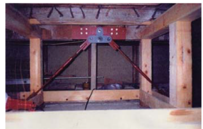
Damper installed in the space under the floorboards
